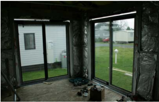
Sliding doors (issue: lock was not equipped)
